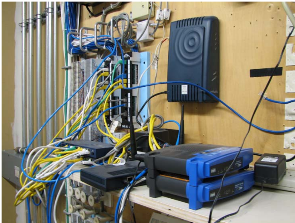
Some end-user equipment located in the third floor IDF. This is located on the opposite wall from the IDF feeder and station cable terminations.
