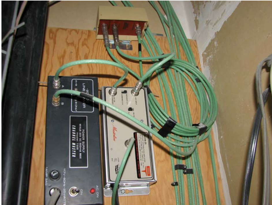
Active equipment (amplifiers) for the coax cables located in the third floor IDF.
