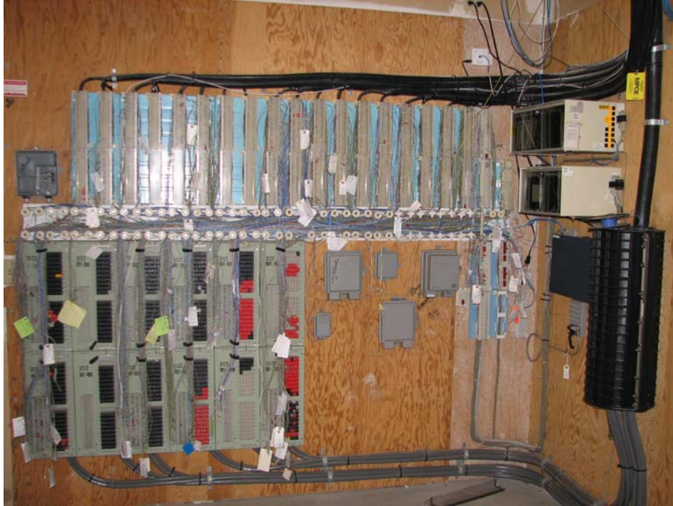
The copper termination from the “street” (LEC). Notice green protection field. Blue field above is for the IDF feeders.
