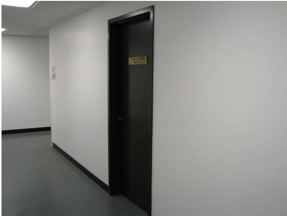
The MPOE location behind the elevators on the basement level.
