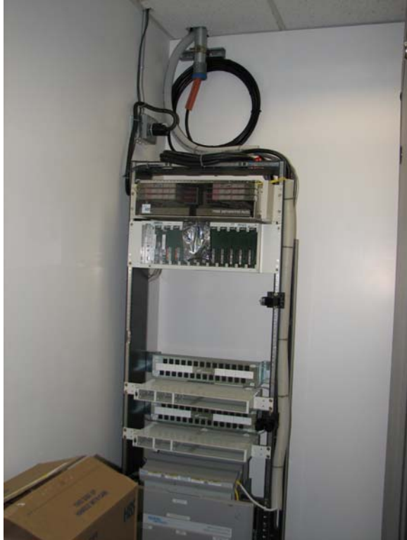
The Optera3400 fiber termination in Suite 100. This feeds through the MPOE and is the only fiber termination for the building, though there is a coil of fiber, without termination, in the MPOE.
