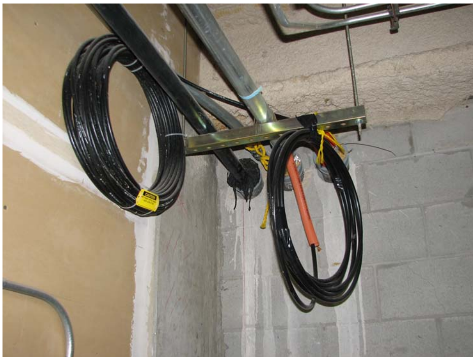
The entry point from the “street” (LEC) for the copper and fiber Telco Facilities cables. Notice fiber coil on left continues the run to first floor – Suite 100. Coil on right ends there and is not terminated.
