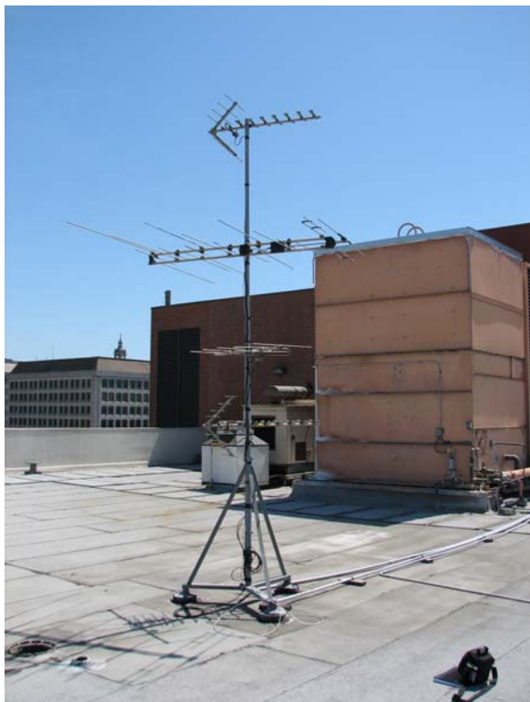
The antennae upright on the roof with multi-service antennae attached. Alfa Tech Cambridge Group
