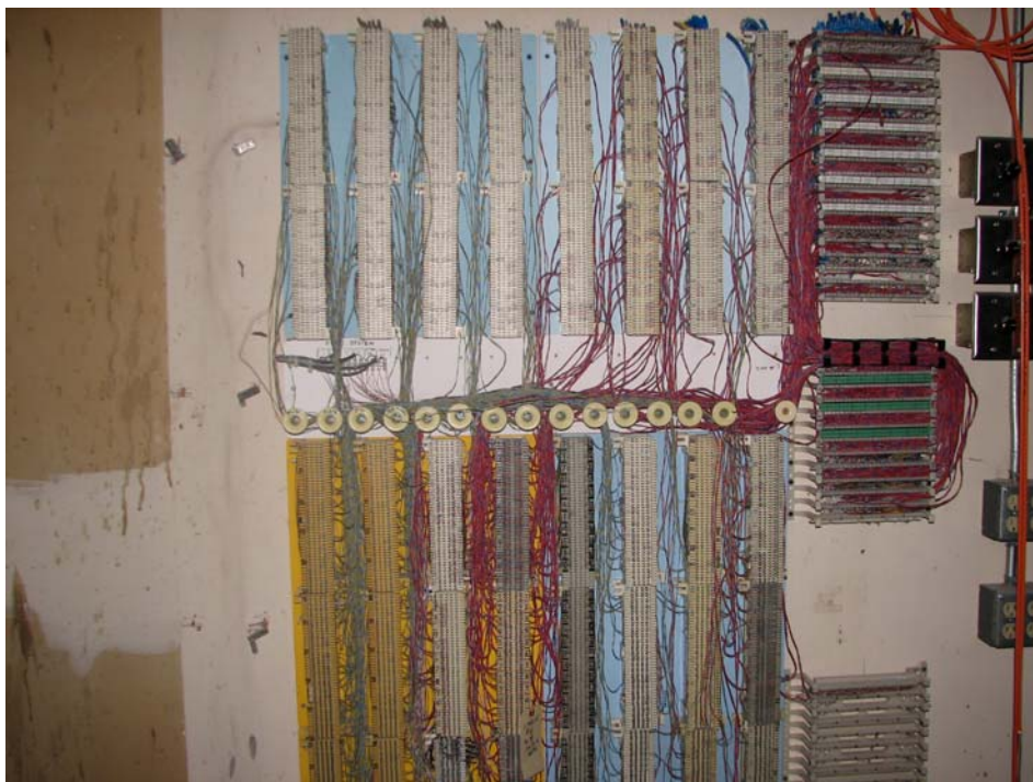
One of the IDFs in the building. The cables have been cut-off above the termination blocks.
